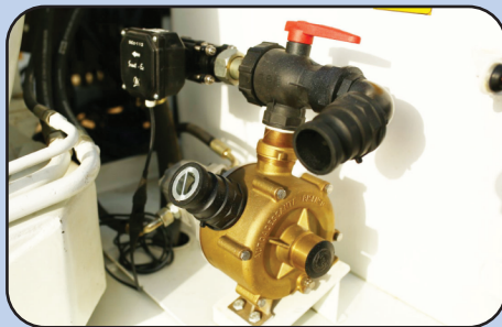
Water Pump and Imported Fittings
